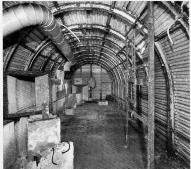
AC plant room. Photo by Nick Catford
